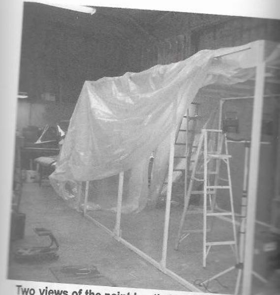
Two views of the paint booth Scott built for the recovery. This view shows the rest of the work area.
